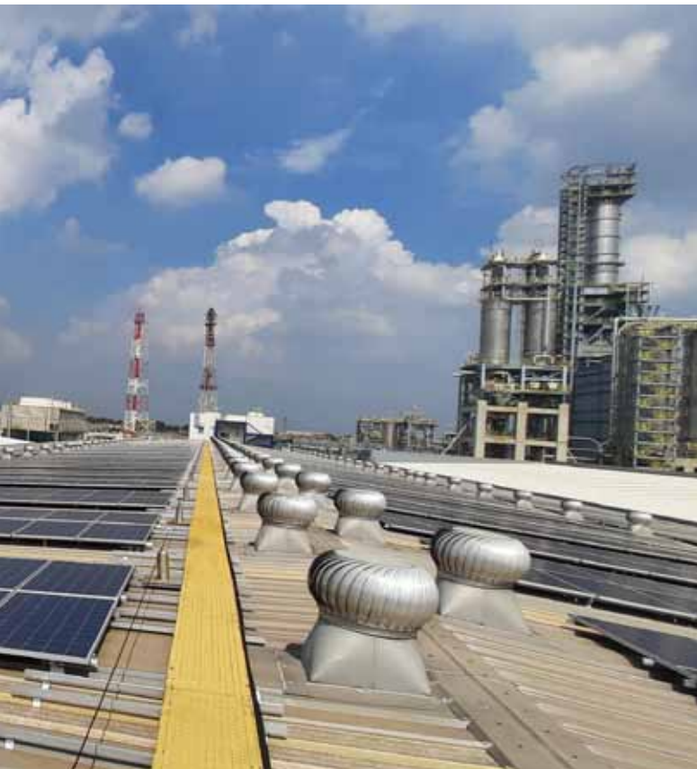
Cross section of solar panel installation located in Chandra Asri office complex.
